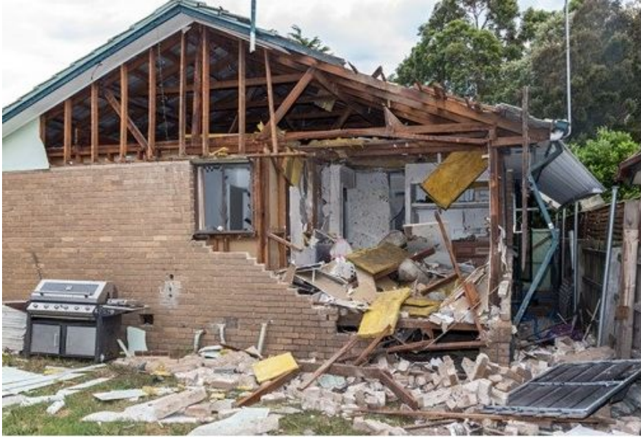
Home in New Zealand, after water heater explosion
